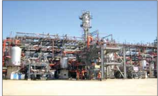
Gas Sweetening & C2+ Recovery Unit
