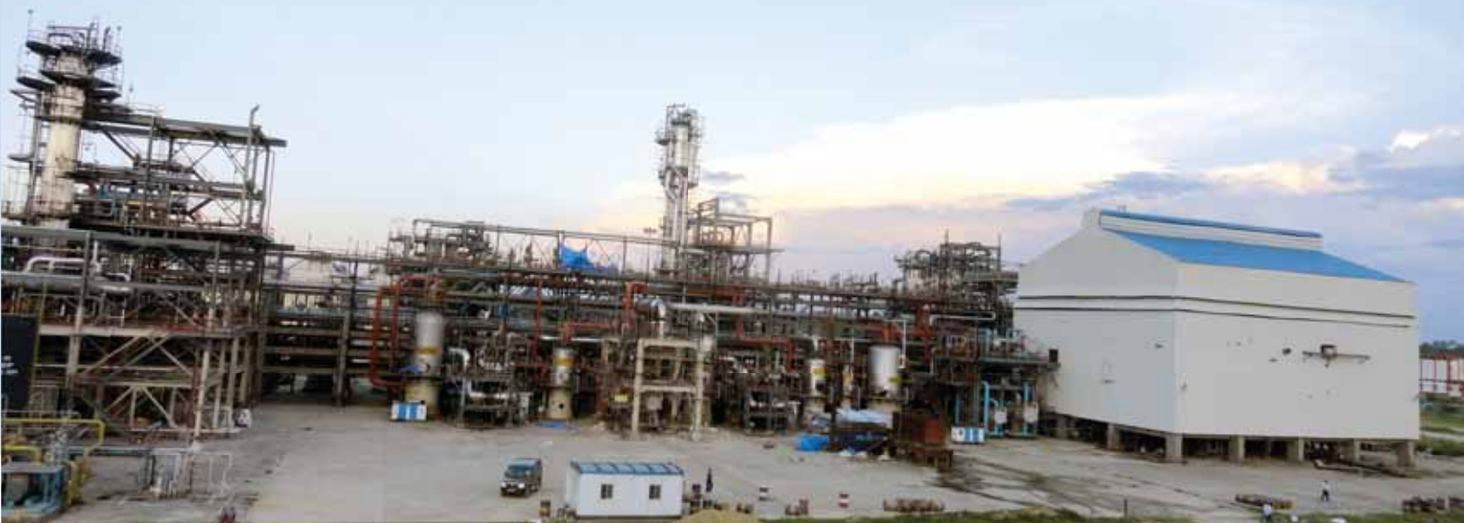
Gas Sweetening Unit
