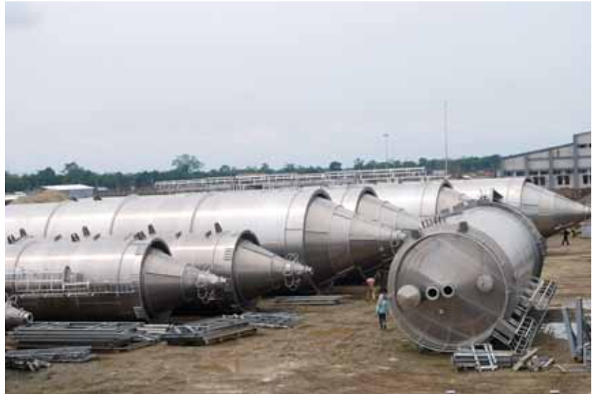
Cyls for the HDPE/LLDPE unit
