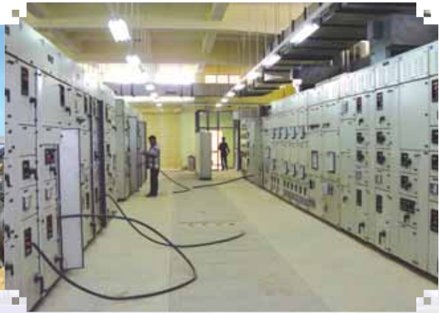
Sub Station Panel Room
