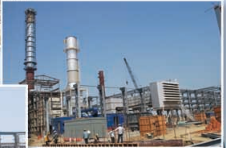
The Captive Power Plant
