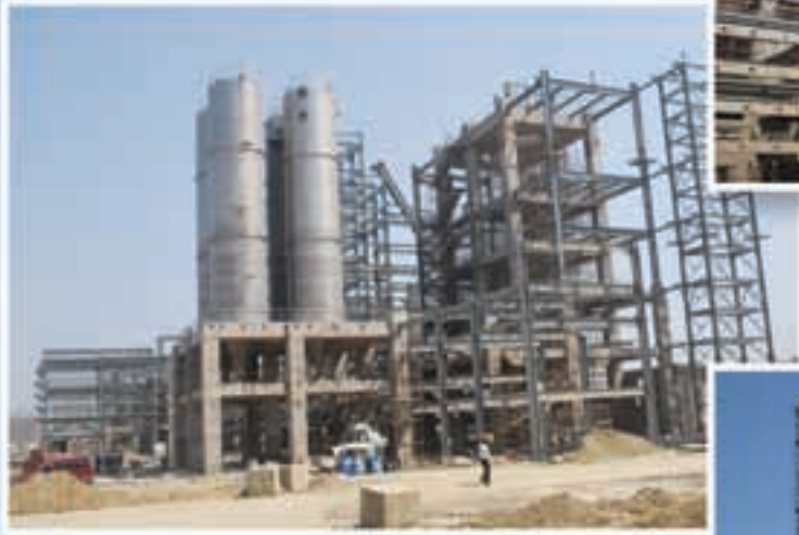
Polypropylene Unit with four Pellet Blending Silos
