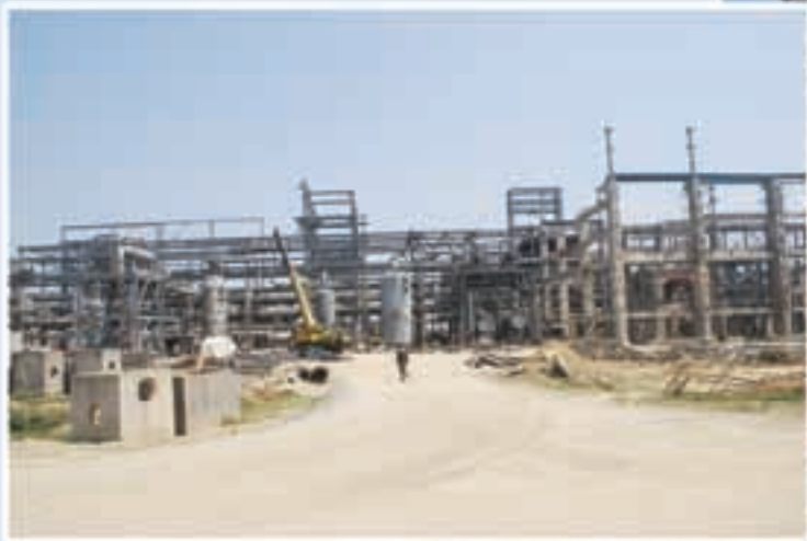
The Ethylene Cracker Unit
